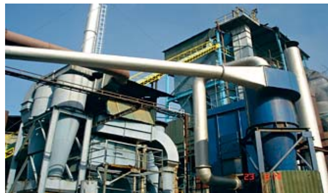
Co-generation plants produce power from agricultural wastes & combustible wastes coming out of manufacturing activity
